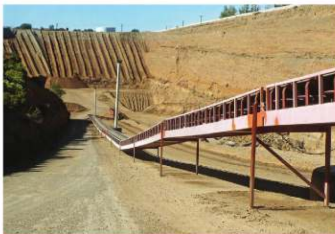
Material is pushed down the slope by a dozer, loaded into a crusher by a loader, and then carried up a conveyor system to the processing plant.
